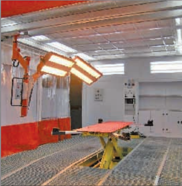
INTERNO PREP STATION CON SOLLEVATORE E LAMPADA AEREA INTERNAL PREP STATION WITH SUSPENDED INFRA-RED LAMP
